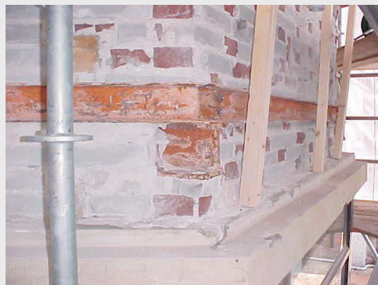
Corroderende stalen frame's
